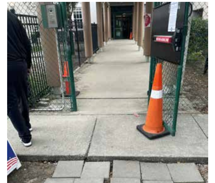
Uneven pavement outside a poll site presents an accessibility challenge for voters with disabilities. Photo by LDF Staff
